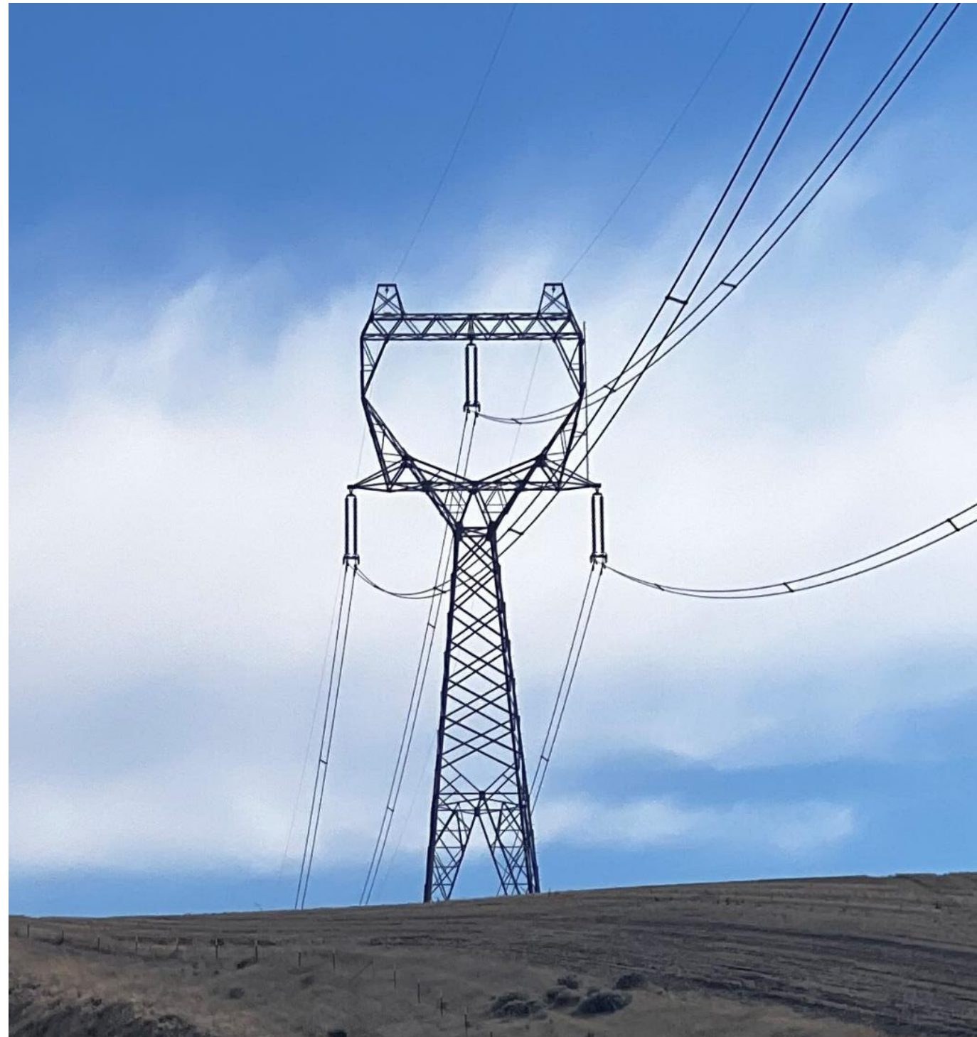
TYPICAL SINGLE CIRCUIT 500-KV TRANSMISSION
